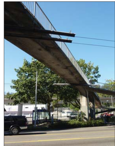
Pedestrian bridge at the intersection of MLK Jr. Way S. and Rainier Avenue S.
