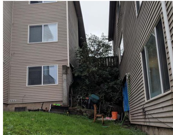
Plate 4. Photo of Rockery at 3416 House
