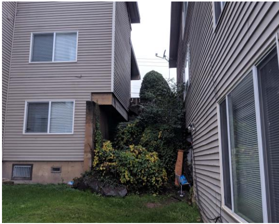
Plate 3. Photo of Rockery at 3410 House
