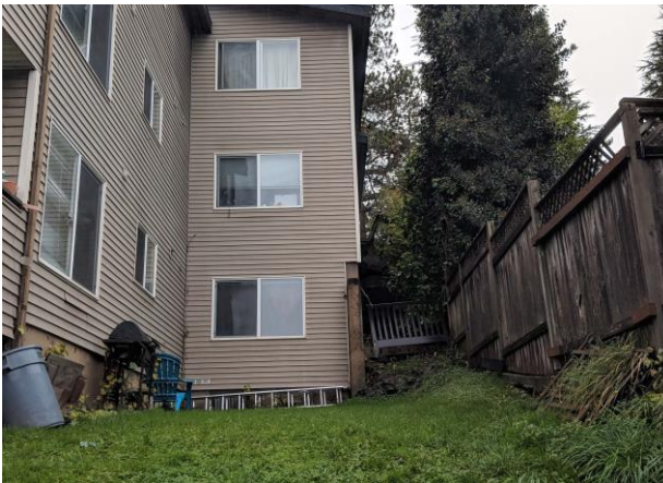
Plate 5. Photo of Rockery at 3420 House
